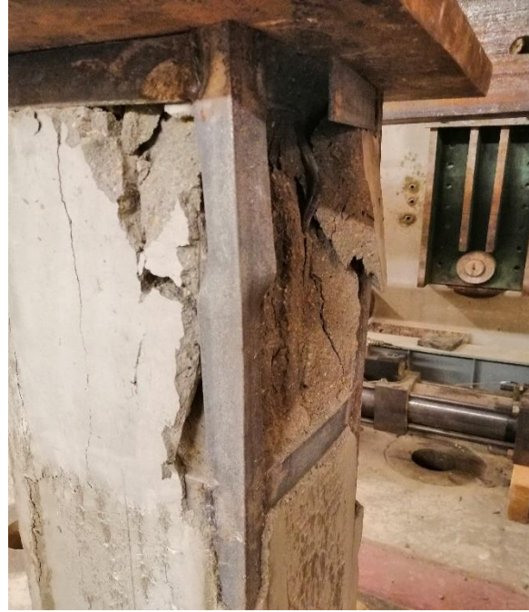
Figure 4-13: Failure of column C52
