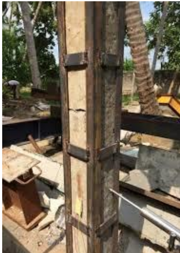
Figure 2-9: Steel jacketed RC column (Amulya, 2010)
