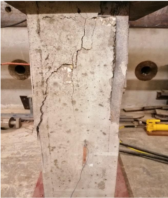
Figure 4-10: Failure of column C41
