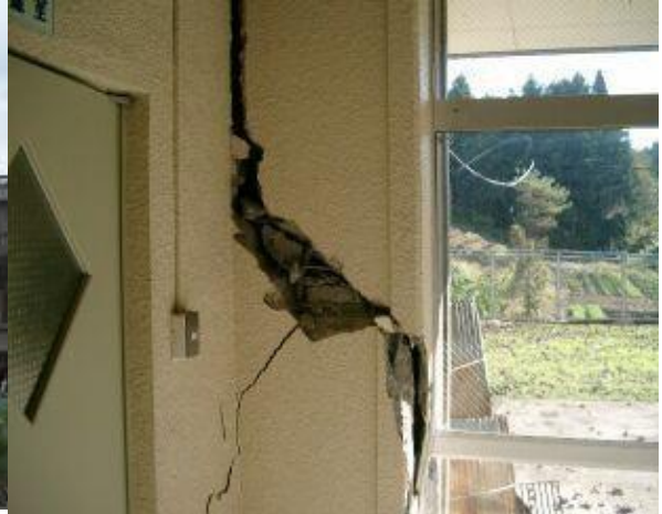
Figure 1-3: Shear Failure in a column ( www.pinsdaddy.com )
