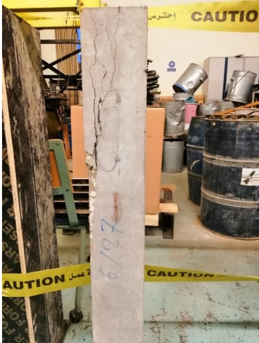
Figure 4-4: Failure of column C11
